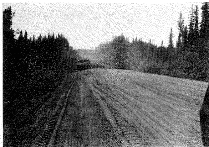
FIG. 4. Liard Highway, early June 1983. Construction in progress south of the Poplar River crossing to repair damage to the roadbed caused by spring runoff.
