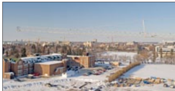
Five construction cranes could be seen working on the University of Saskatchewan campus during the winter of 2010.
